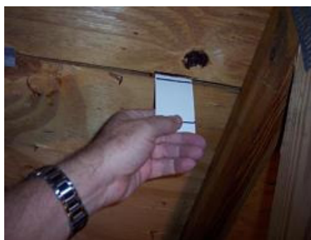
Using heavy paper to measure roof deck thickness (click image for larger version)
